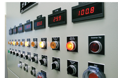
Local Operating Panel
